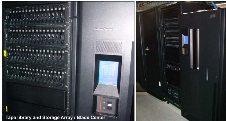
Tape library and Storage Array / Blade Center
